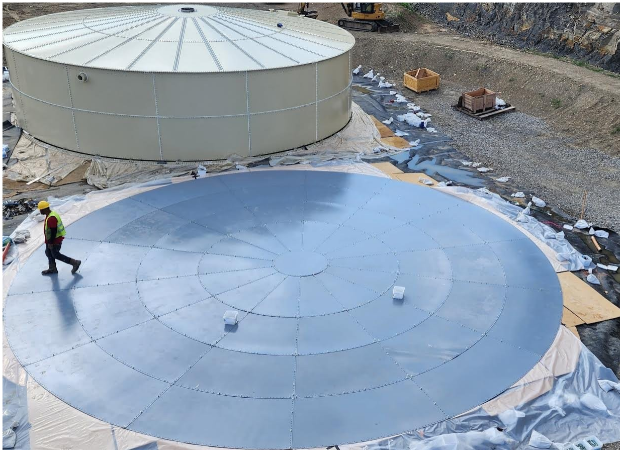
Photo 9 — Bolted steel roof on a completed FBE tank (rear) with the bolted floor of a second tank laid out on its foundation pad (front). Both roof and floor are assembled from sealed, bolted lap joints exactly like the shell.
