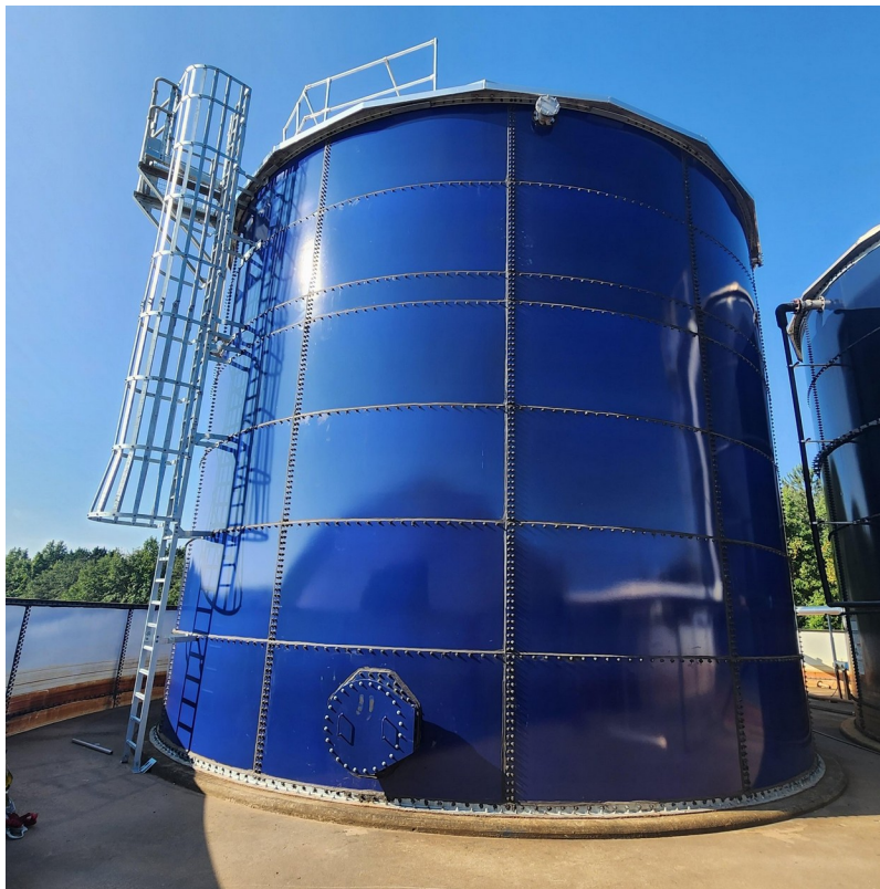
Glass-fused-to-steel bolted tank with exterior caged ladder and roof handrail
